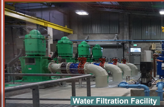
Heidi Lansdowne Intake Facility on Bridge Creek
