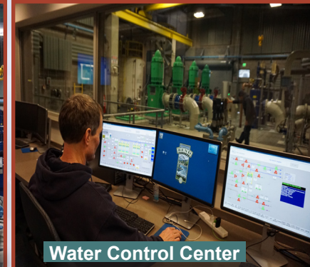
Water Filtration Facility
